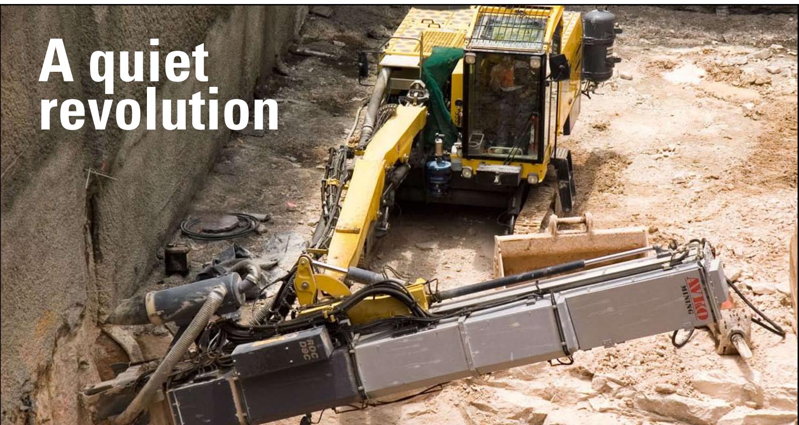
Smart, silent type ... the Atlas Copco ROC D9C Silenced Smart Rig at work on a section of the $A2 billion Brisbane North-South Bypass Tunnel project.
